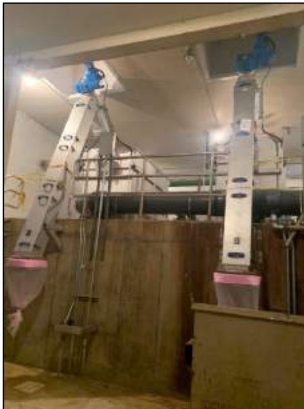
FIGURE 4-3: HEADWORKS DRUM SCREENS
