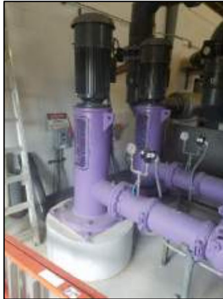
FIGURE 4-8 EFFLUENT LIFT STATION
