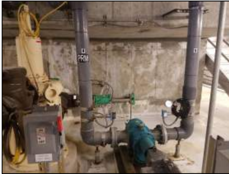
FIGURE 4-6: MBR PERMEATE PUMP
