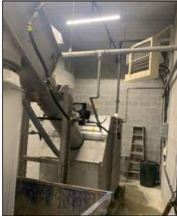
FIGURE 4-4: SEPTAGE RECEIVING STATION
