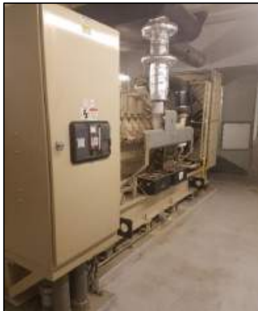
FIGURE 4-11: MBR STANDBY GENERATOR
