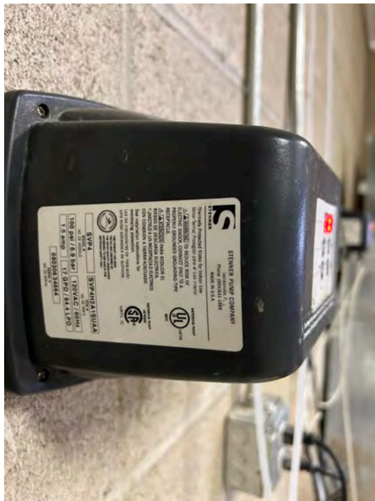
Photograph 14: Chemical injection pump specs
