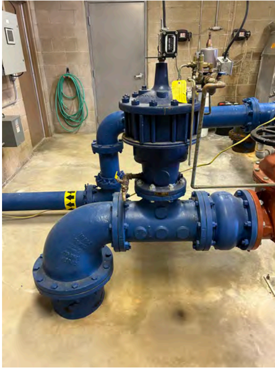
Photograph 5: Well #2 entering the wellhouse
