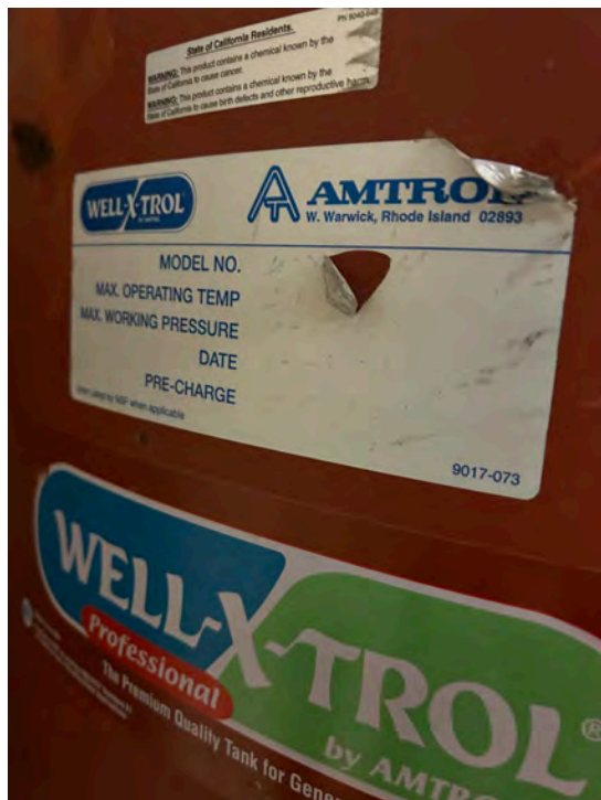
Photograph 17: Pressure tank tag - Well Xtrol; WX-4
