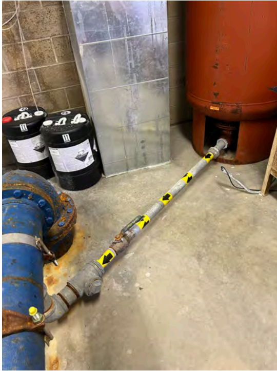
Photograph 15: Pressure tank isolation valve and union
