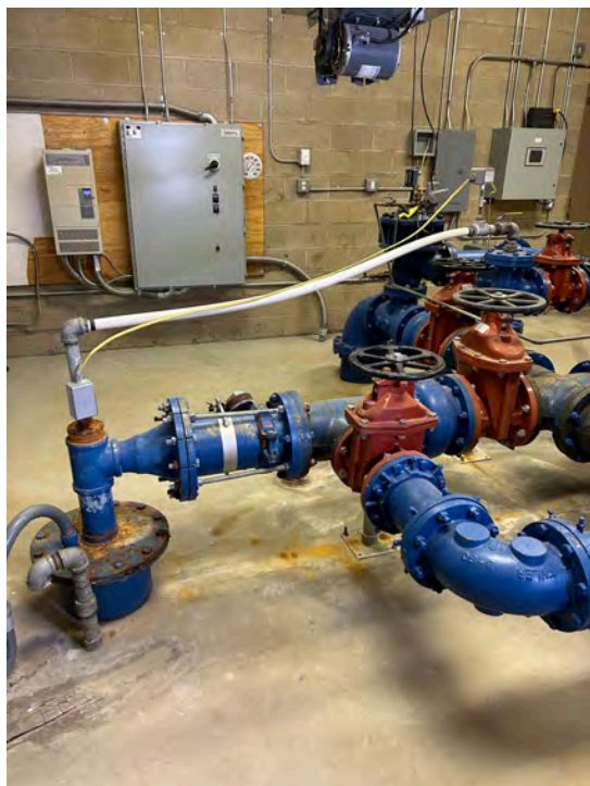
Photograph 2: Well #1 wellhead and piping
