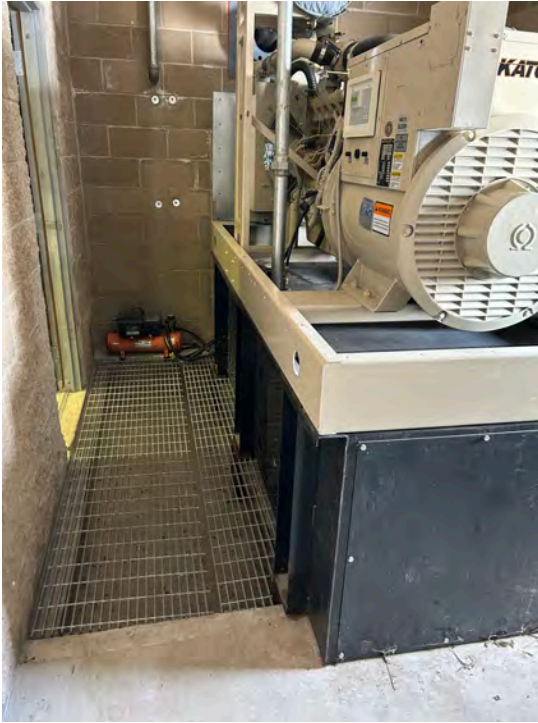
Photograph 19: Backup generator with secondary containment
