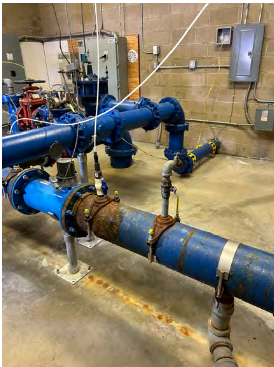
Photograph 8: Chemical injection on pipe to distribution
