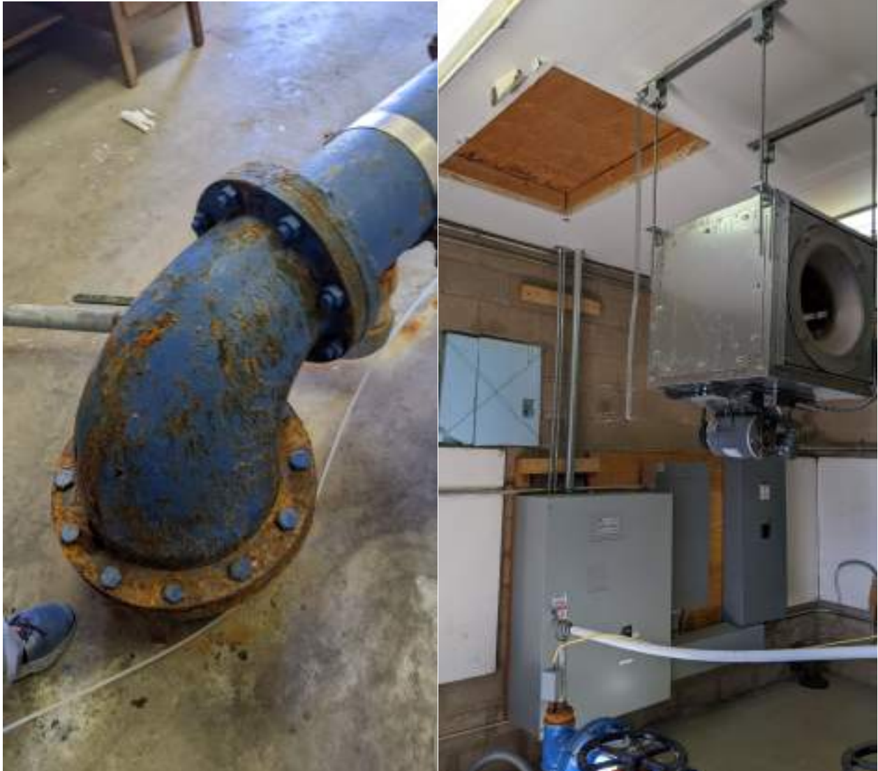
FIGURE 3-11: HAWKS BAY (RUST, ROOF LEAK, AND UNUSED EHASUT FAN)
