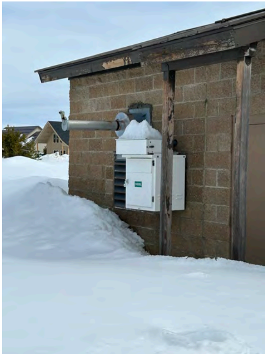
Photograph 24: Exhaust for generator
