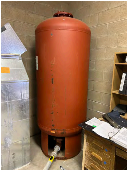
Photograph 16: Bladderless pressure tank
