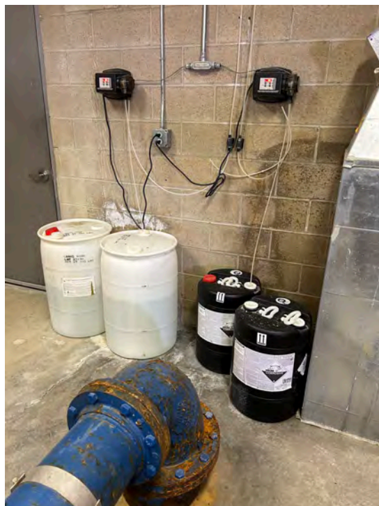
Photograph 11: Chemical injection setting
