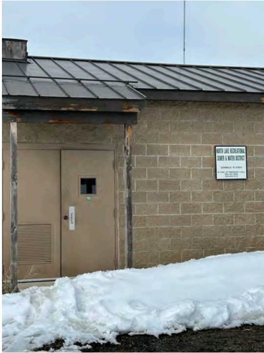
Photograph 25: Wellhouse door - lockable; emergency contact info on placard
